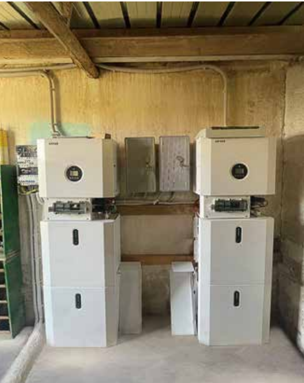
09 Residential ESS Project in Italy
