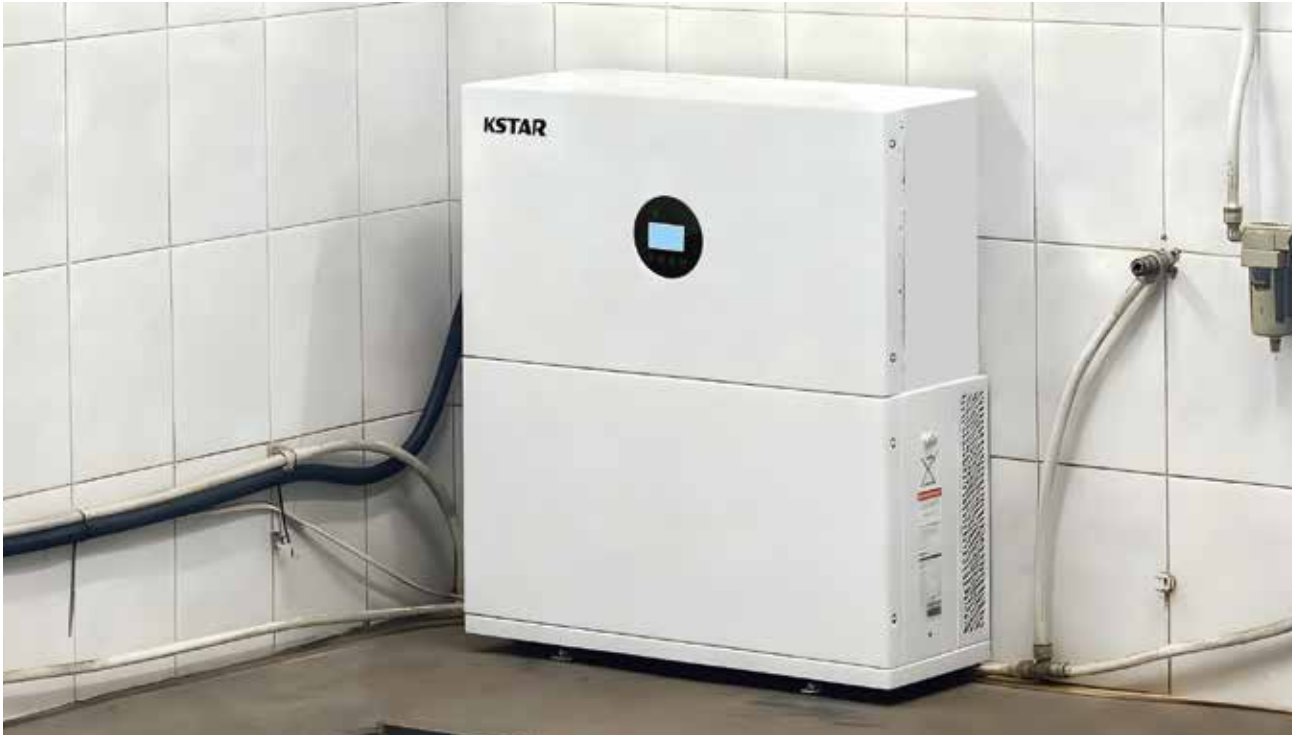
06 Residential ESS Project in Ukraine
