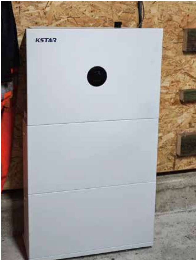
02 Residential ESS Project in the Netherlands
