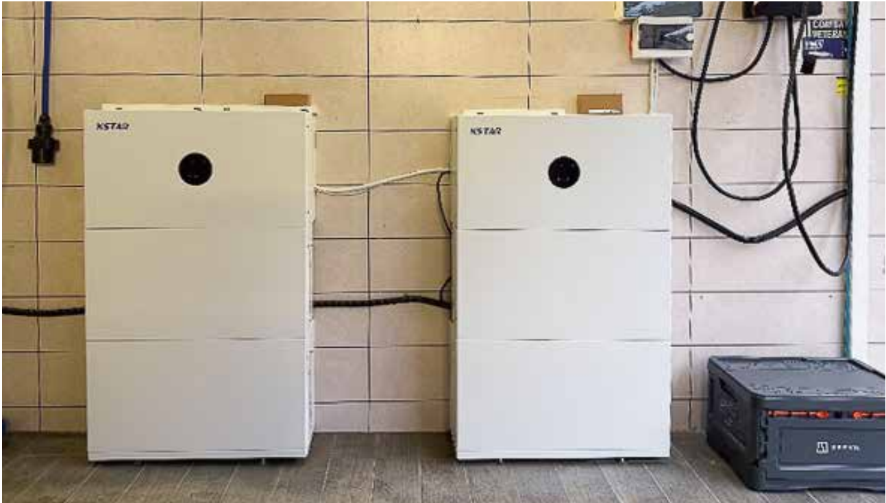
05 Residential ESS Project in Ukraine
