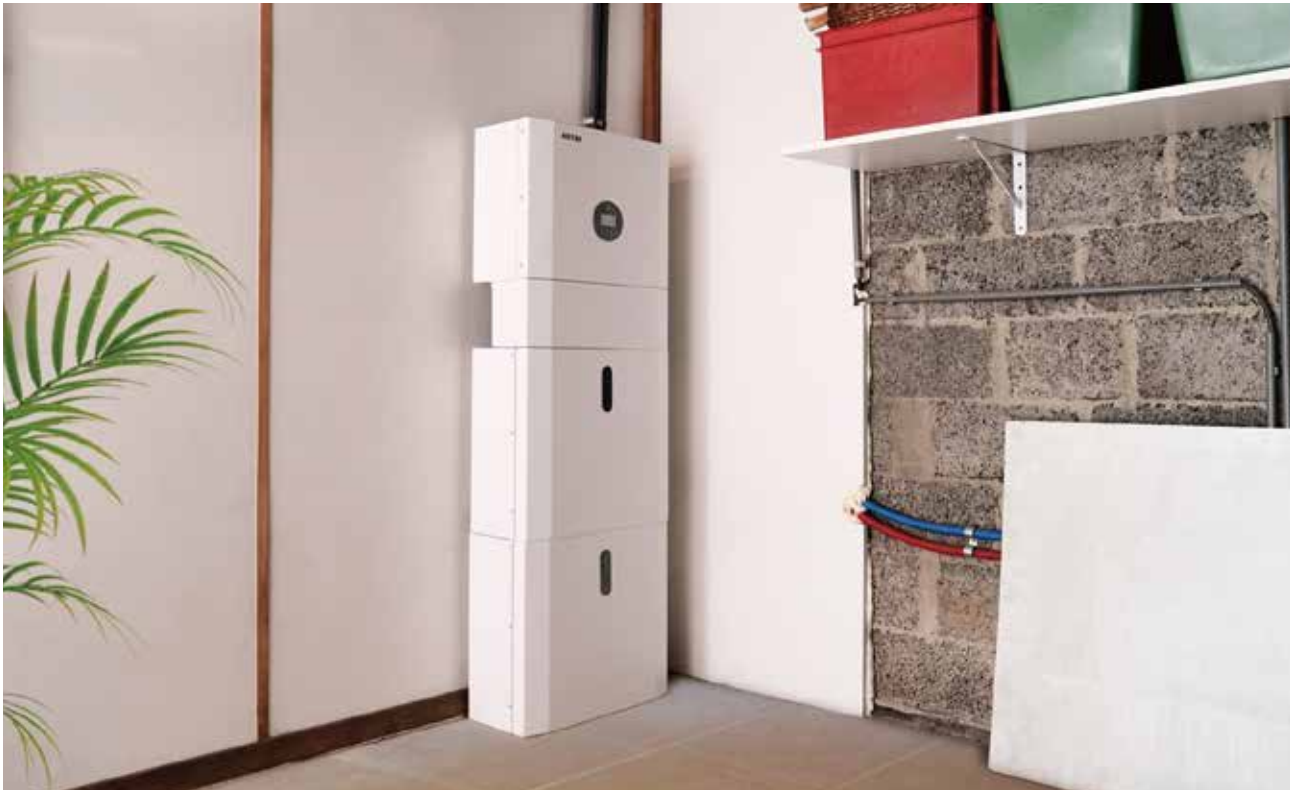
10 Residential ESS Project in the Netherlands
