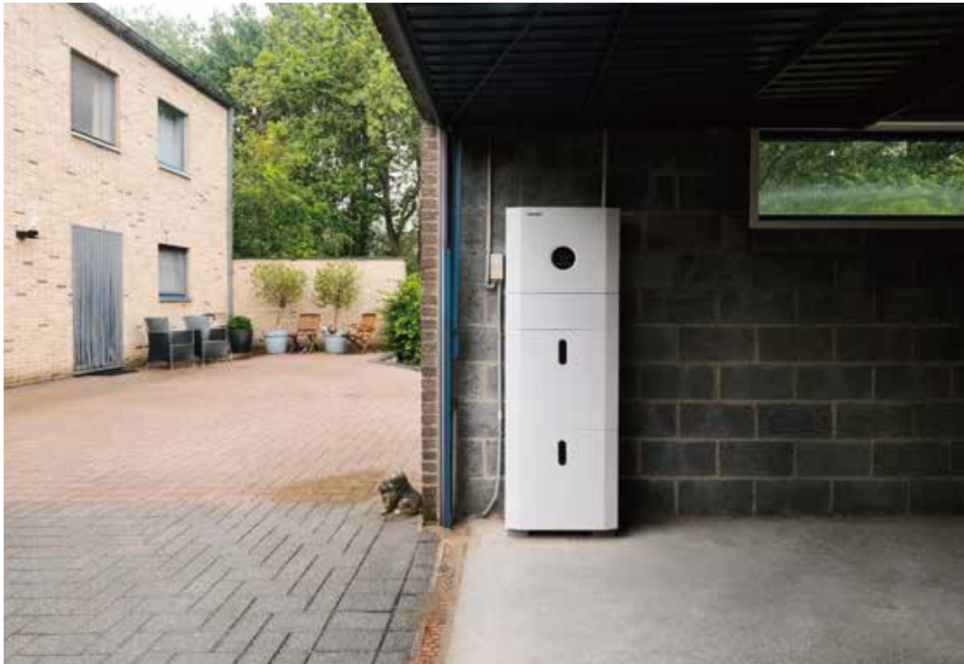
15 Residential ESS Project in Belgium
