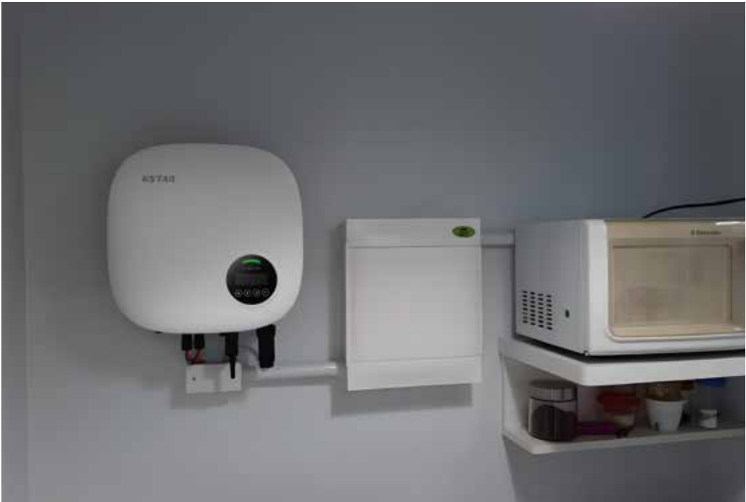
14 Residential Solar Project in Brazil
