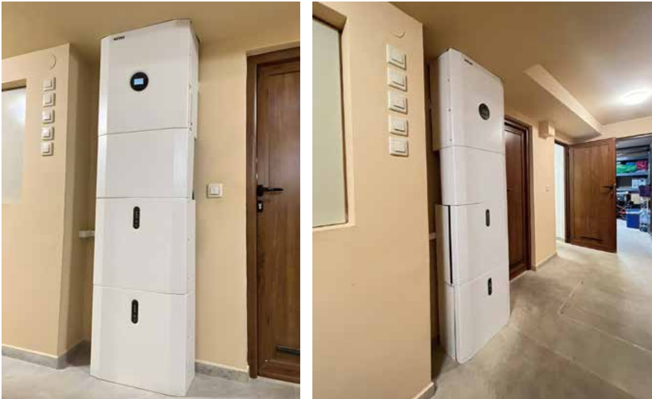
07 Residential ESS Project in Bulgaria
