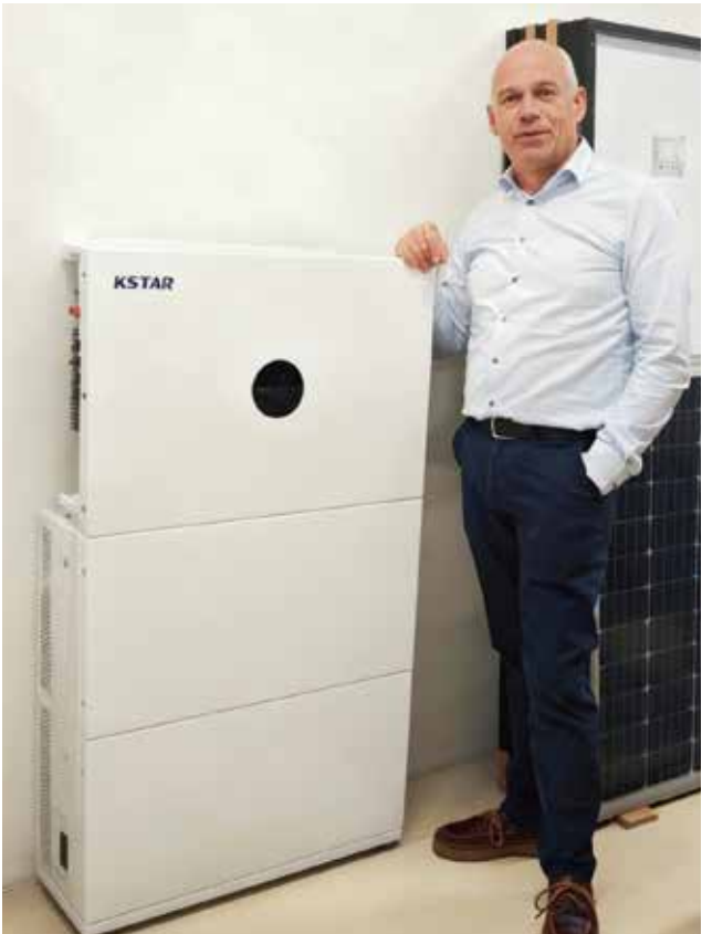
03 Residential ESS Project in the Netherlands
