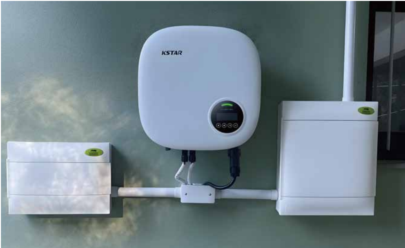
11 Residential Solar Project in Brazil
