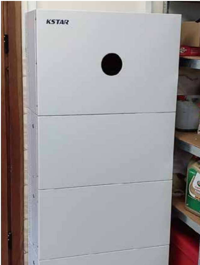
01 Residential ESS Project in Lithuania
